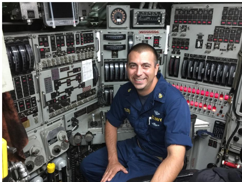
Chief Flores at the Ballast Control Panel on board USS Albuquerque on its final voyage before decommissioning in October 2015
